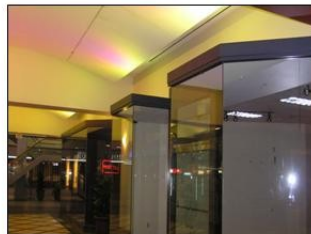
The original 400-watt high intensity lights giving off illumination on the ceiling above the windows seen in this photo, will be replaced by 85-watt florescent lamps, which provide an energy savings as well as good illumination.
